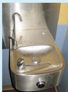
Bellevue Union School District in Santa Rosa, CA, retrofitted their fountains to add a bottle filler next to the traditional drinking fountain. The District also installed wall-mounted cup dispensers to provide cups to students to use if they did not bring a reusable water bottle. 2
